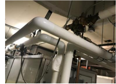
Chilled Water Makeup w/ RPBP Bypass Connected to Strainer!
