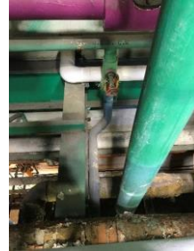
Domestic Water Backup – Condensate Tank – Taken From Catwalk
